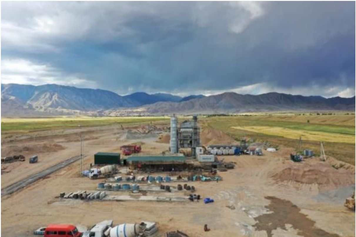
Figure 20: Asphalt concrete plant at the production site (km 148+630).
