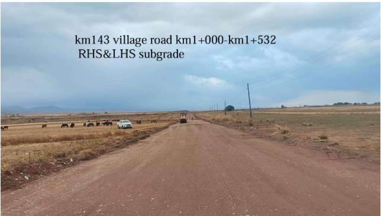
Figure 10: Subgrade on the section km 1+000 – km 1+532 of the additional rural access road to the village of Kuyruchuk (km 143).
