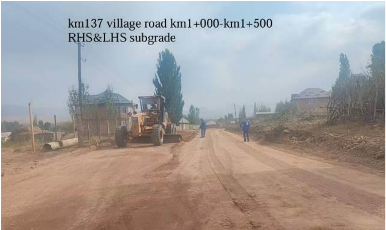
Figure 9: Subgrade on the section km 1+000 – km 1+500 of the additional rural access road to the village of Kyzart (km 137).
