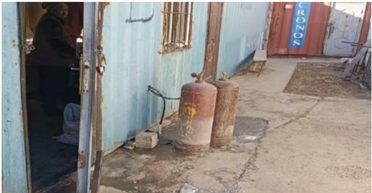
Figure 37: Violation of gas cylinder storage
