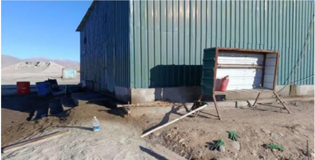
Figure 36: Incomplete fire shields
